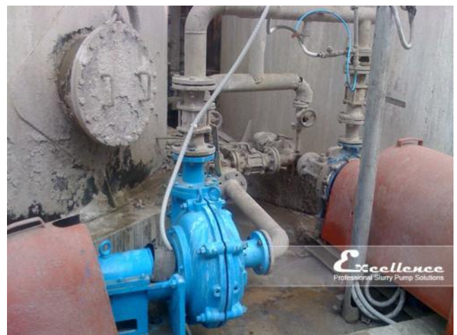
50EZ-A50 in Mid-East Sodium Silicate Plant
